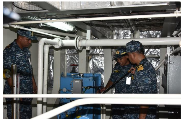
Commander Submarine inspecting the engineroom of Submarine tugboat.
